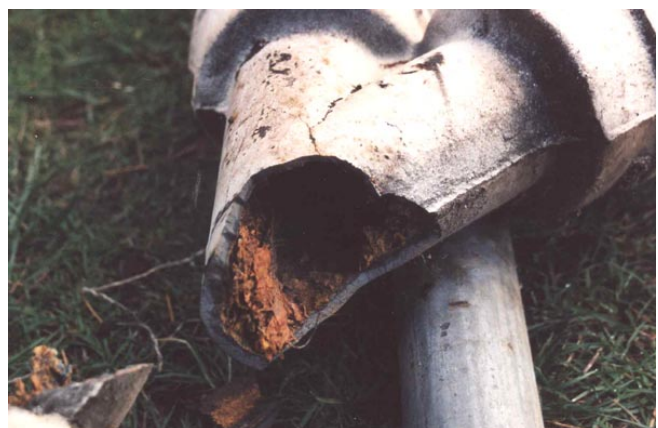
Galvanized pipe rusts from the inside out making it difficult to detect problems.
